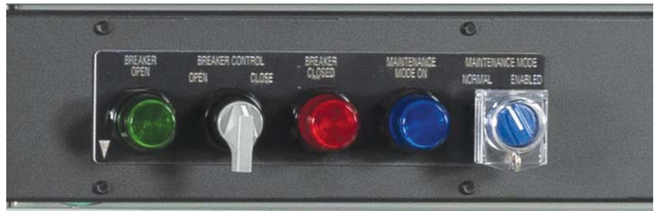
Devices Mounted on Secondary Terminal Compartment Door
