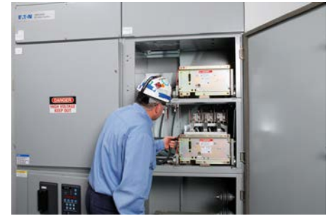
Arcflash Reduction Maintenance System
