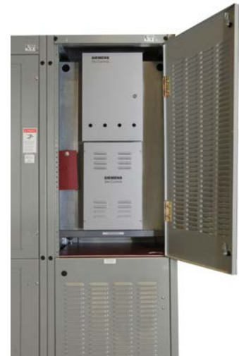
Building Management System
